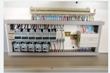
Siemens electrical components and PLC control
