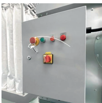
8. E-Control cabinet Schneider switch
