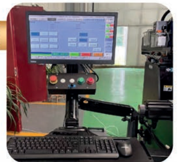
Advanced Control System
